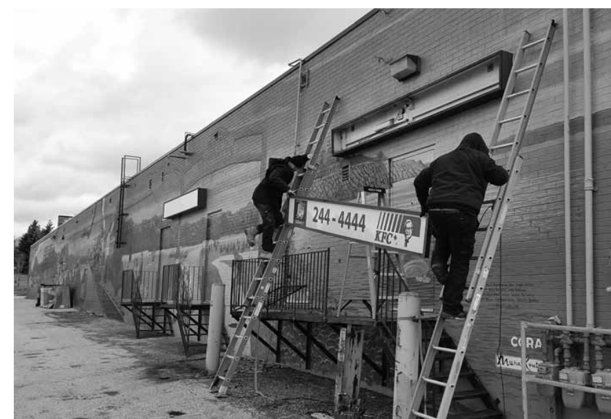
Paul Stiel, electrician and owner of KS Electric Co., and Dwayne Hawkins remove the KFC sign from the mural in early April.
